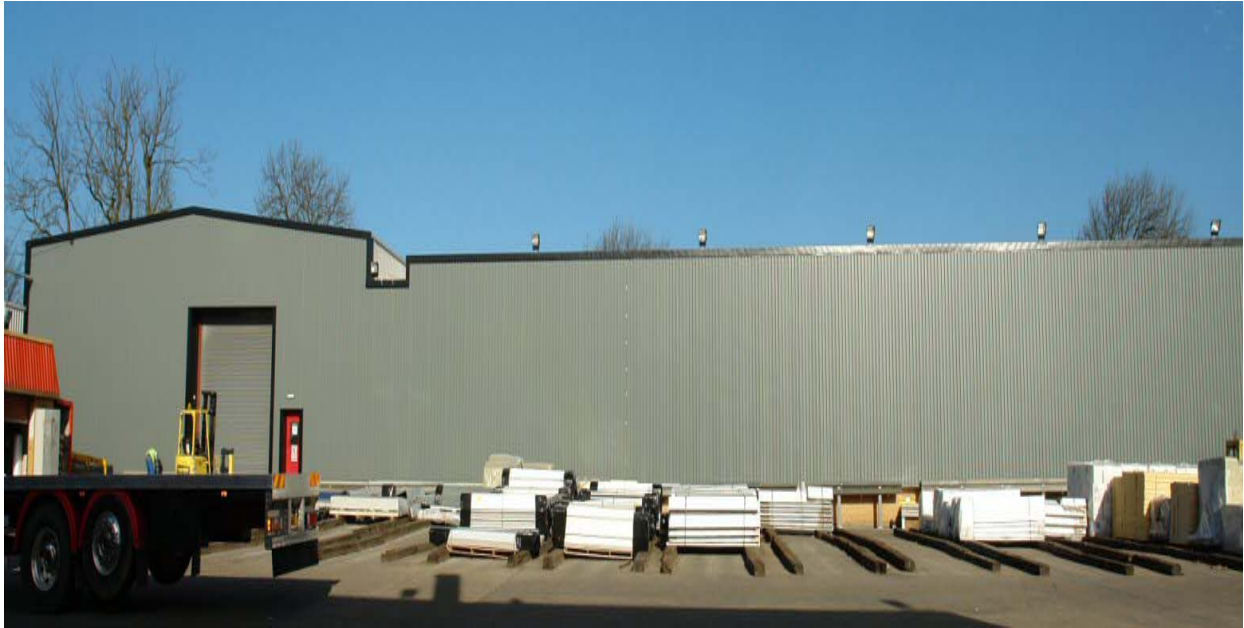
South East Elevation over cladded with metal SolarWall™ system
