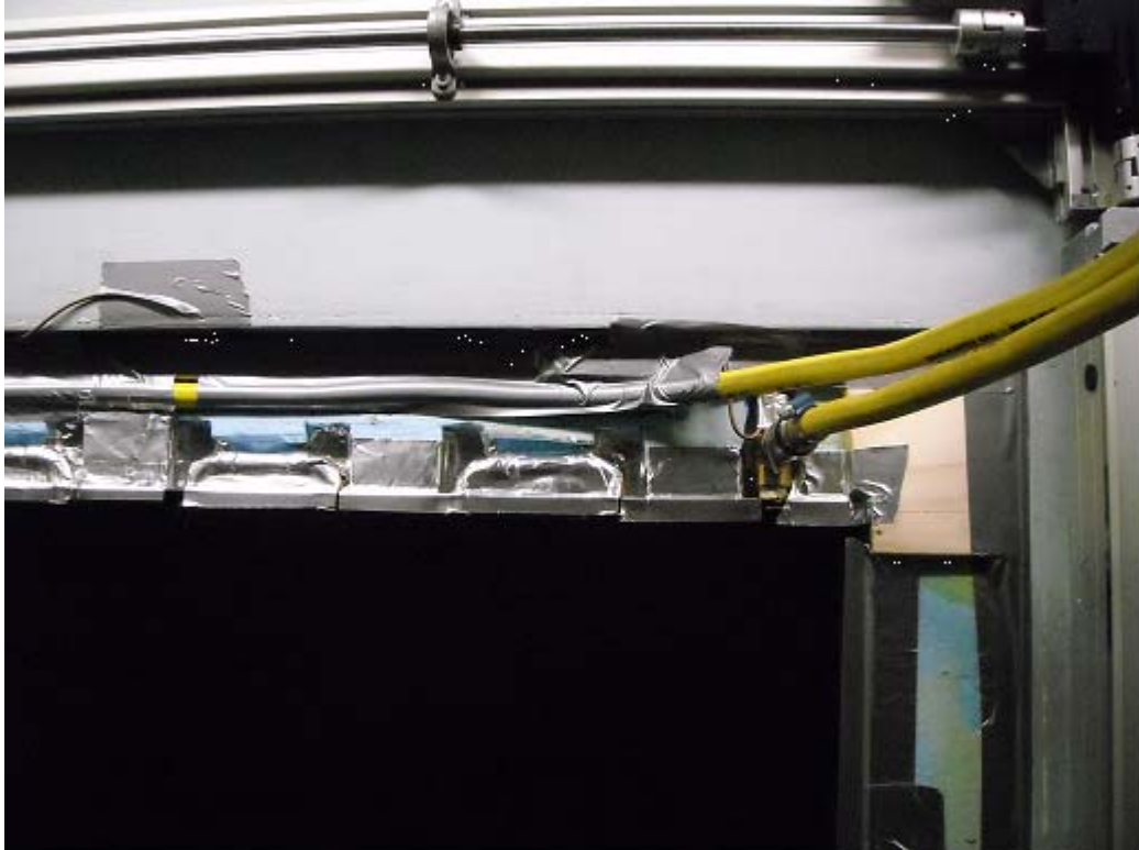
Figure 12. Copper pipes connected to liquid circuit (water in test case). By-pass circuit was used to balance mass flow rate of the collector
