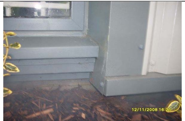
Figure 11 Picture showing leakage from window jamb
