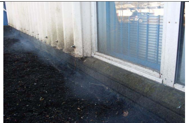
Figure 7: Picture showing leakage from asbestos cladding and dwarf wall interface
