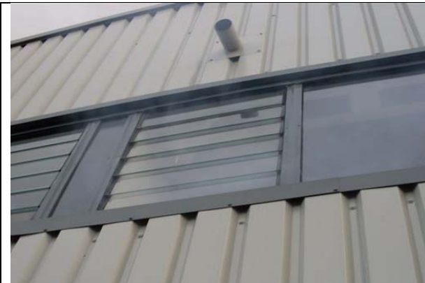
Figure 10: Picture showing leakage from window interface
