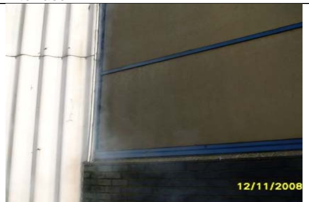
Figure 9: Picture showing leakage from window jamb
