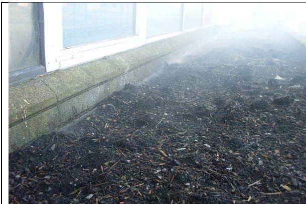
Figure 6: Picture showing leakage from window sill
