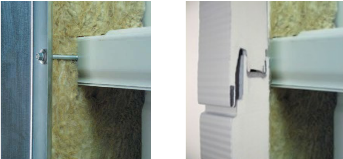
Figure 1.2 Re-cladding with additional insulation layer (Rockwool: “Steelrock”, left), overcladding using steel sandwich elements (right)
