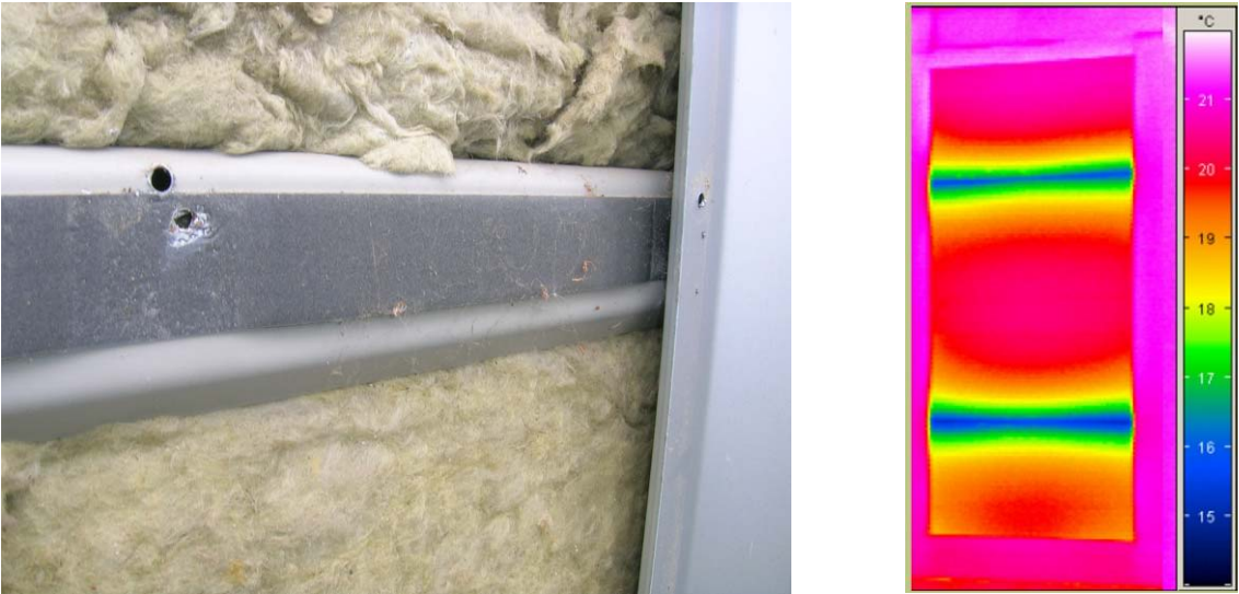
Figure 1.1 Existing state of cassette wall (left), IR-survey cassette wall in Hot-Box (right)
