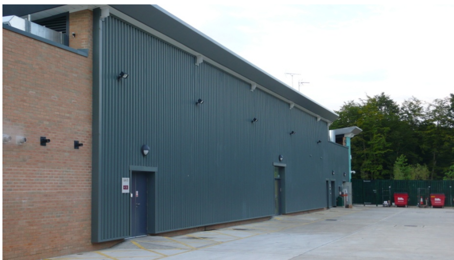
Figure 4 SolarWall® TSCs installed on the south wall of Beaconsfield service station (UK), where the TSC preheats the ventilation air for the food court
