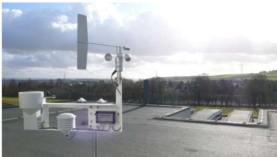
Figure 13 Weather station as viewed from the monitored facade
