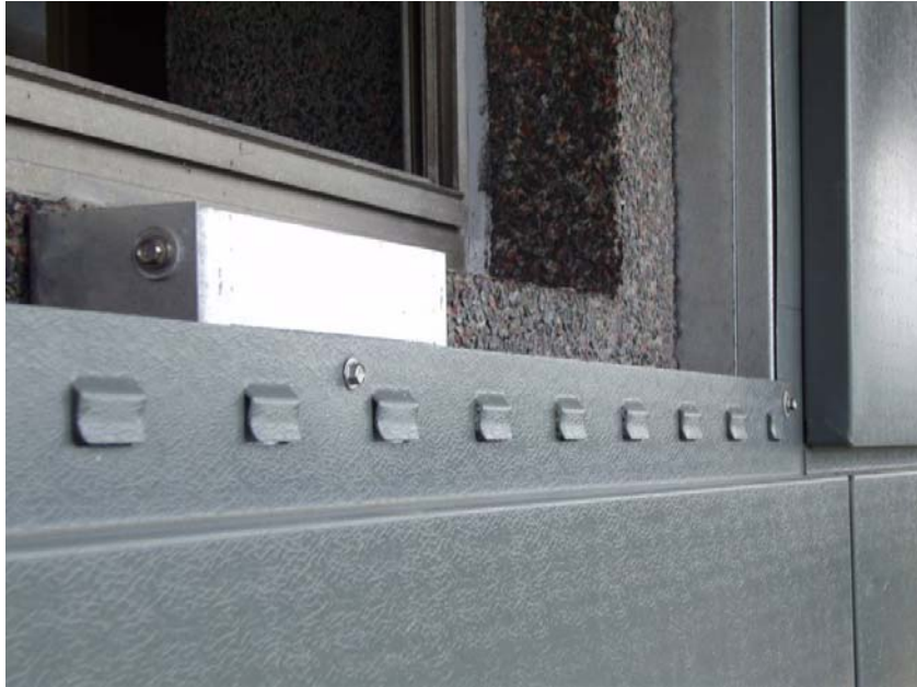
Figure 10 Horizontal joint detail between the panels showing the top hat section behind
