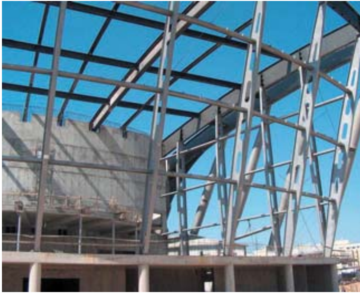
Figure 3. Scanning is used for surveying cladding substructure attachment points. Image courtesy: Mabat
